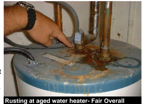
Rusting at aged water heater- Fair Overall
