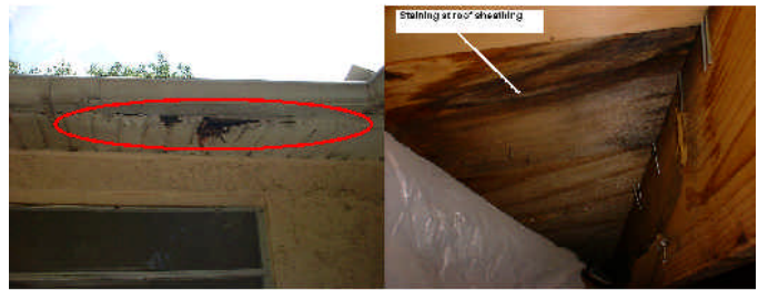
Damaged Overhang/Roof Problems/Leakage
