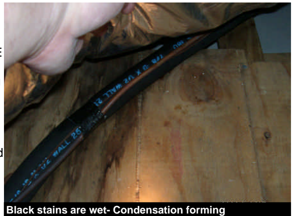
Black stains are wet- Condensation forming
