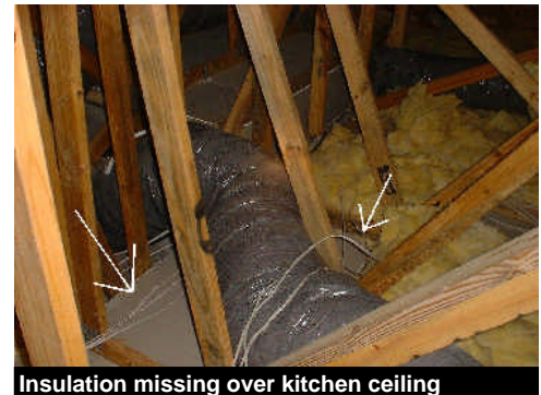
Insulation missing over kitchen ceiling
