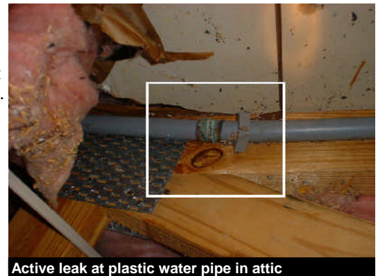
Active leak at plastic water pipe in attic
