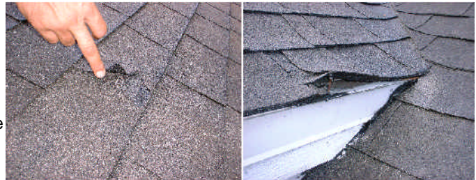
Protruding staple - Uplifted edge flashing
